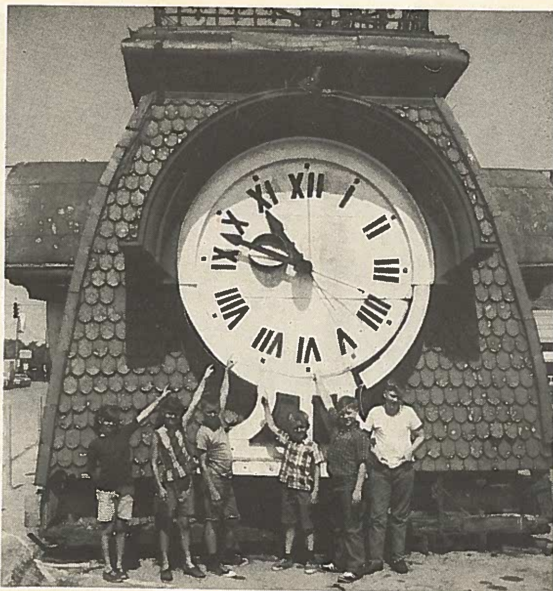
GRANBURY YOUNGSTERS HAVE HAD A GOOD TIME LOOKING OVER THE HUGE CLOCK - DOME WHICH ORDINARILY TOPS THE GRANBURY COURT HOUSE. IT WAS REMOVED ABOUT THE MIDDLE OF JUNE IN ORDER TO MAKE MUCH-NEEDED REPAIRS. PICTURED IN THE PHOTO ABOVE ARE: (LEFT TO RIGHT) SHARLA, SHERRY, AND SHELDON FRENCH; MACK CAMPBELL, CRAIG HILLMAN AND RANDY FREDERICK.
