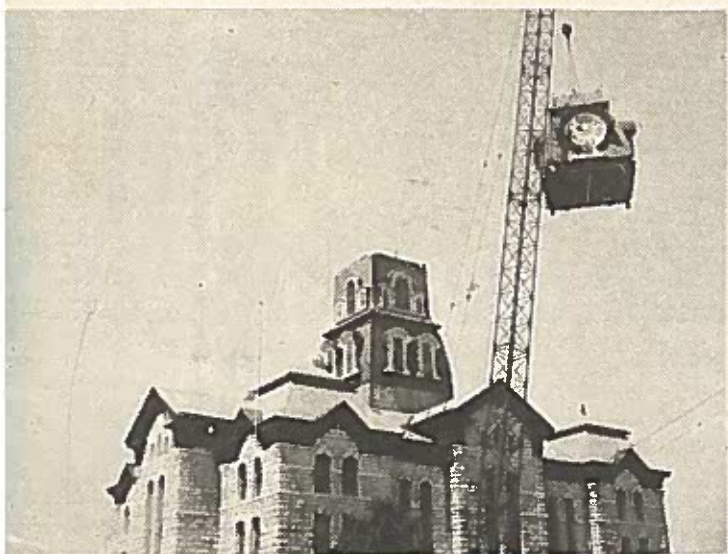
AN ENORMOUS CRANE PLUCKED THE DOME FROM HIGH ATOP THE GRANBURY COURT HOUSE AS RESIDENTS OF THE CITY LINED THE SQUARE TO WATCH THE UNUSUAL SIGHT.
